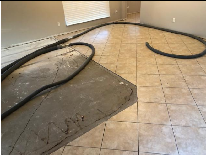
Photo 3: Overview of HEPA vacuum hoses laid out to help collect dust – vacuums kept outdoors
